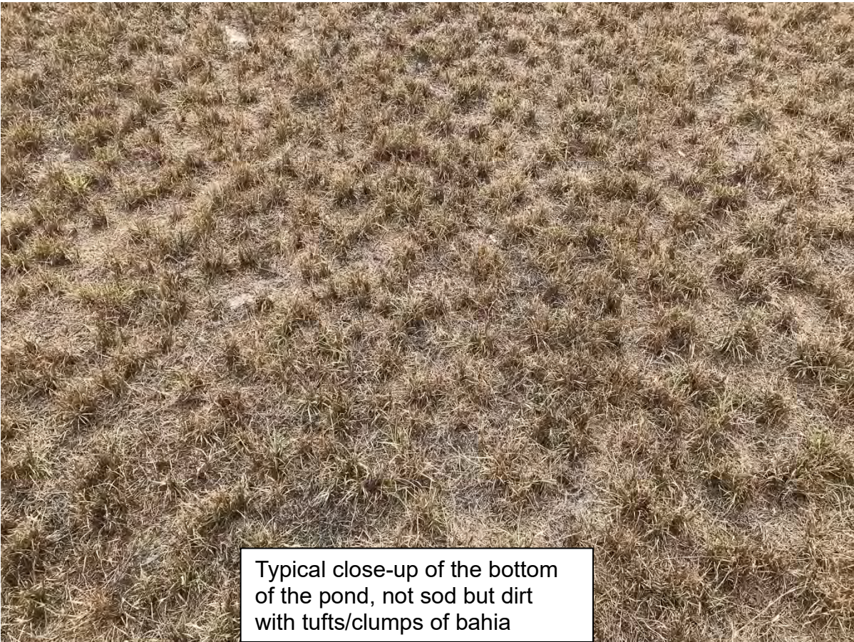
Another nearby inlet to the east, there must be dirt almost to the top of the inlet with weeds coming out of the inlet
